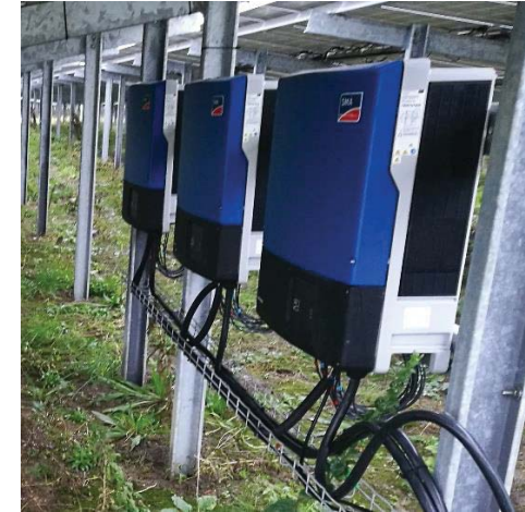
Photo 3 Example string inverters
