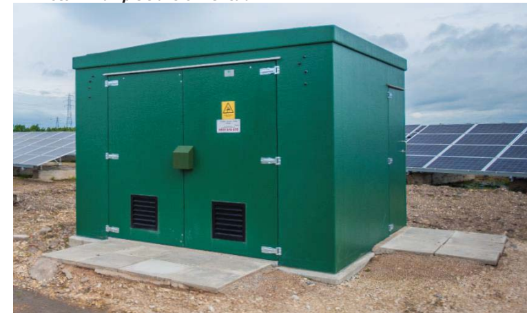
Photo 4 Example transformer cabin
